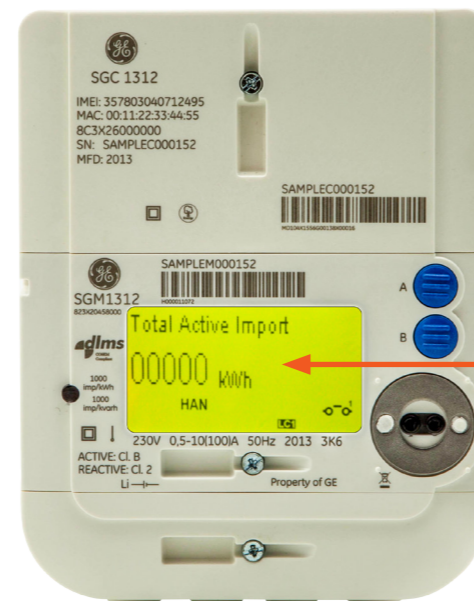
GE electricity meter
